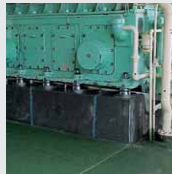
Gas engine on concrete
